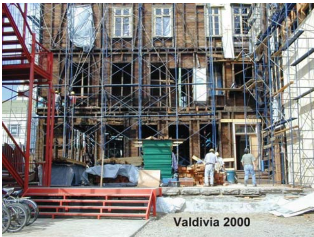
Fig. 5 The remodeling of the Schuster Hotel in 2000, which houses CECS in Valdivia today
