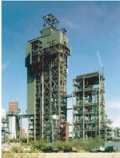
Fig. 8.1. HTW plant in Berrenrath, Germany
