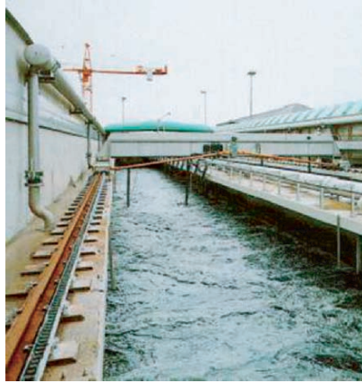
Fig. 8.63. By injecting \text{FeCl}_3 into the sludge, dissolved phosphate precipitates from the waste water
