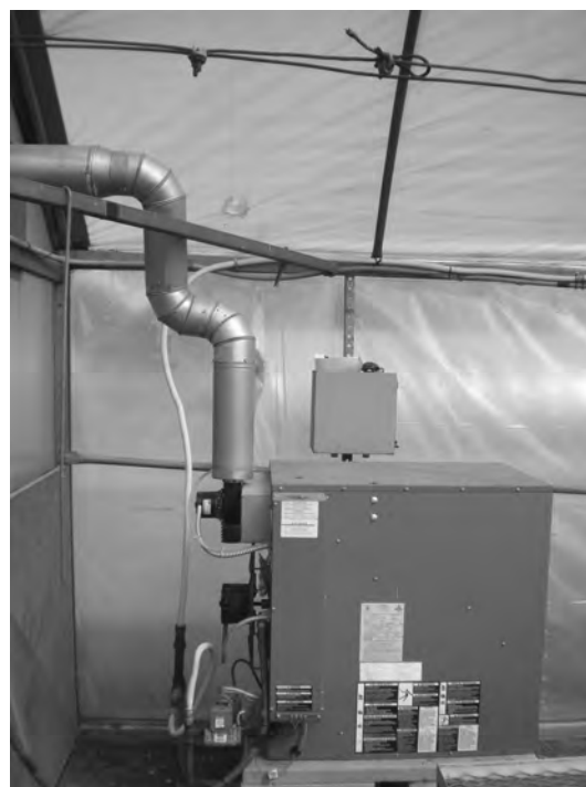
Fig. 11.1. A natural-gas-fueled greenhouse unit space heater. Notice the heater is well ventilated to the outside.
