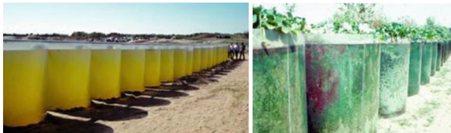
Figure 6. Eco-machines treating septage containing EPA priority pollutants, Harwich, MA (Image: John Todd).
