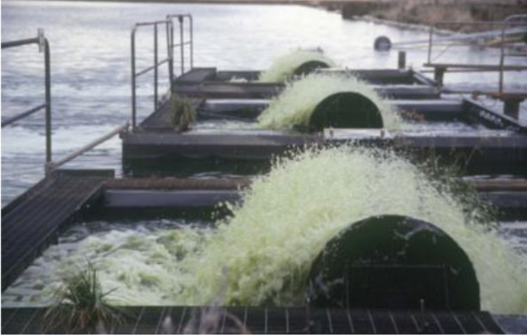
Figure 2. Aquaflow Group Inc. integrated municipal wastewater treatment facility.
