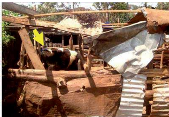
Figure 11. Collapsed iron sheet roof and sides in one of the zero-grazing units evaluated. Both the roof and side timber are broken and collapsing. Yet cows are still housed inside (arrow).
