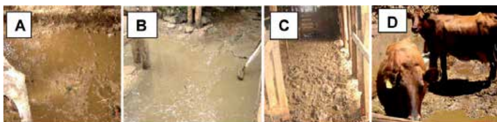
Figure 15. Slurry accumulated in animal facilities. Picture A shows slurry in an earthen floor. Picture B shows slurry in concrete floor. Picture C shows slurry and narrow walk alley. Picture D-Despite slurry accumulation on parks, the cows in this unit were clean because the cubicles had good clean bedding of sawdust, which meant the cows never lay on the slurry.
