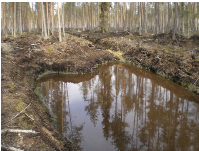
Fig. 17.3 A sedimentation pond constructed to stop soil erosion from a drainage area (Photo: Leena Finér)
